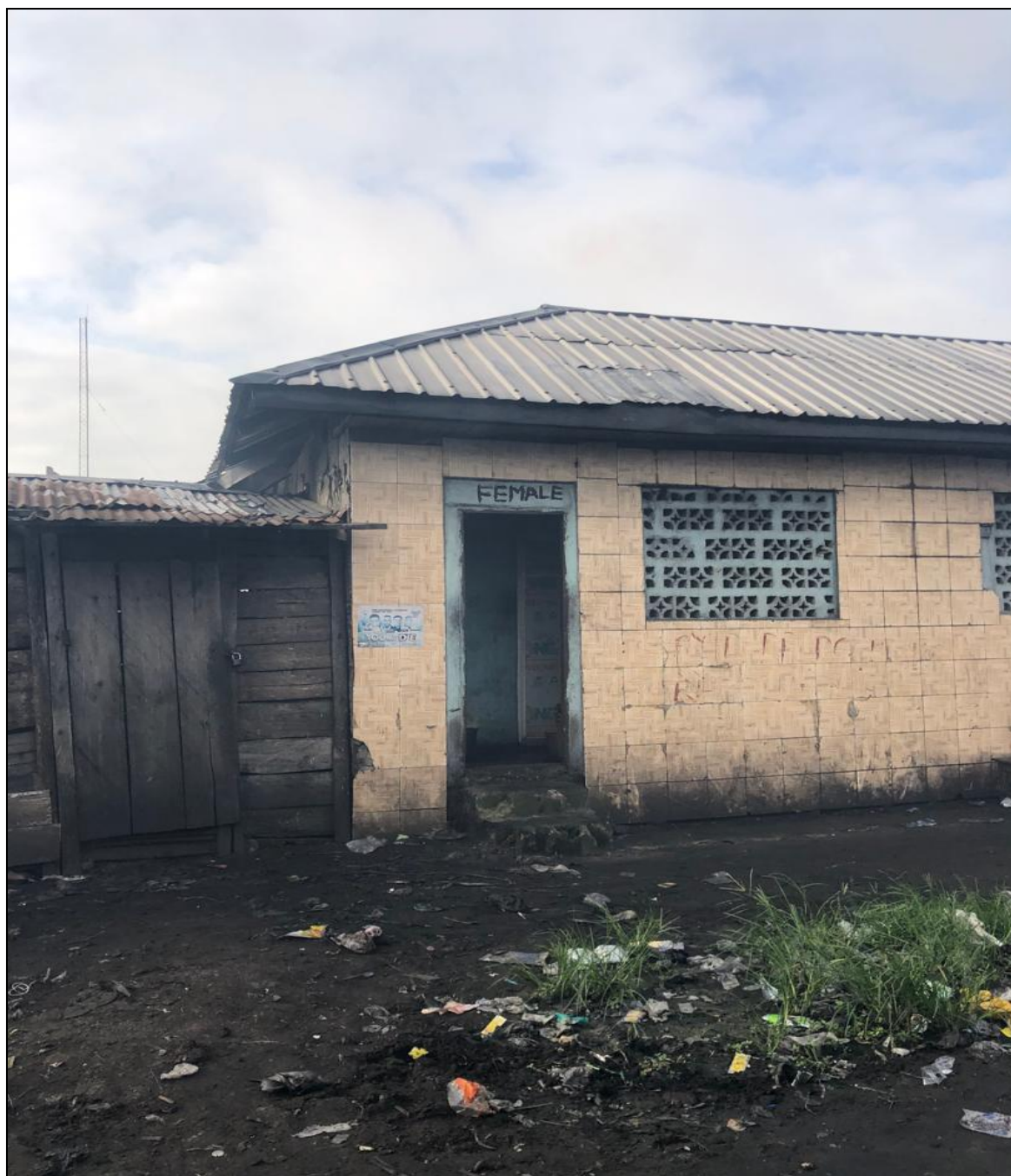
Plate 2 Abattoir Toilet filled with trash and weeds
